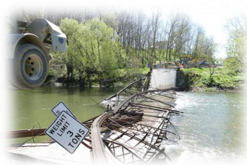
(Courtesy Truckers Report: 30-tonne truck on 3-tonne weight bearing bridge)
